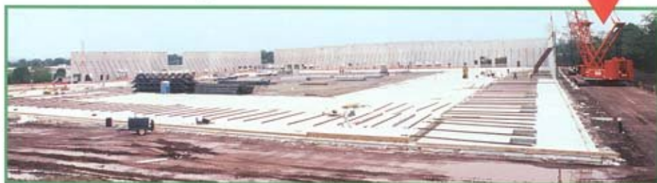
Tilt-up concrete construction is growing in popularity in the Northeast. Shown above is Appalachian Insulation Supply's 200,000-square-foot warehouse under construction in Elizabethtown, PA.
